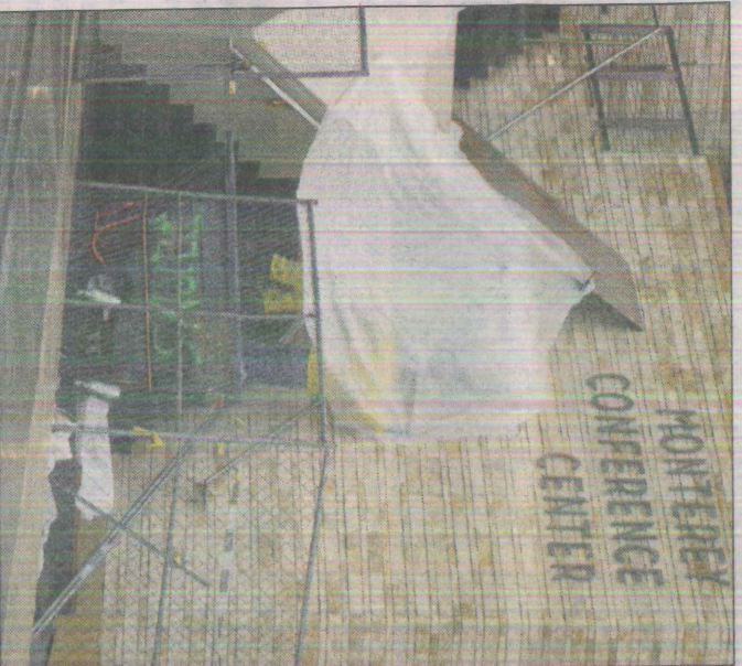
Workers use a plastic tarp to stay dry while working on the outside of the new Monterey Conference Center during a heavy rain shower.
